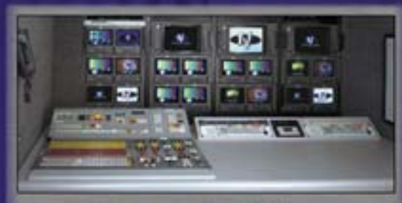
TV-1 Control Room
